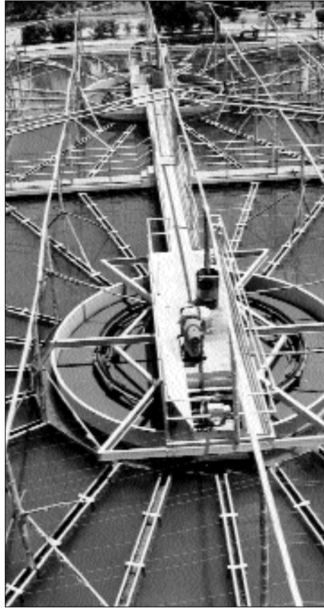
As an emergency measure during the eruption of the Pichincha volcano in Ecuador, in 1999, temporary coverings were installed to protect the water treatment plant from ash-fall.
