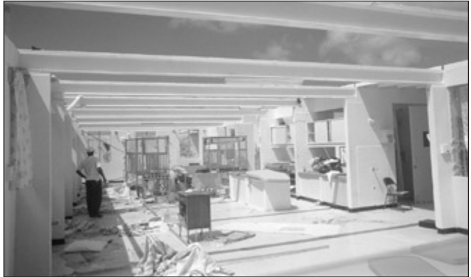
A paediatric ward was made roofless during a hurricane because of the inadequate strength of rafters and their connections. (Photo Tony Gibbs)
