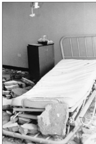
Plaster ceilings should be checked for vulnerability to falling in earthquakes. (Photo PAHO)
