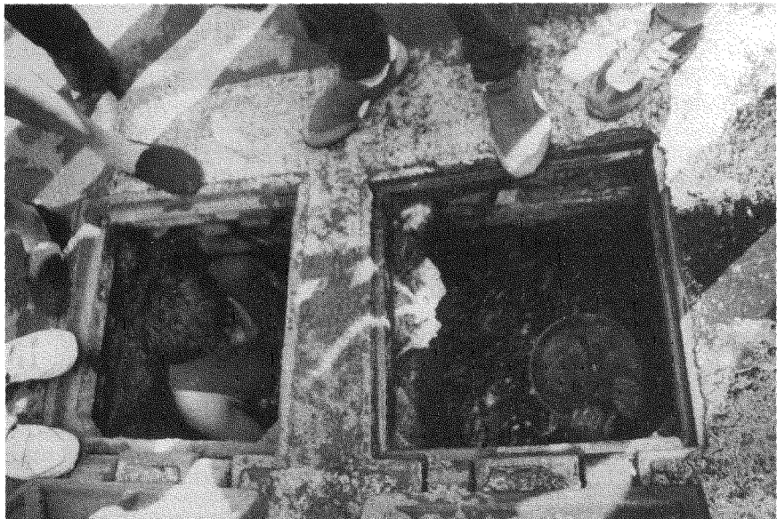
Fig. 18.2. Unsafe break-in into the main water pipe following the earthquake in Mexico, 1985.
